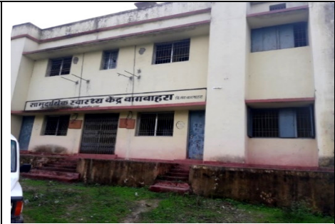
(Date:10/07/2017) Residential quarters at CHC Bagbahra lying vacant since October 2014 for want of electricity and water supply.
