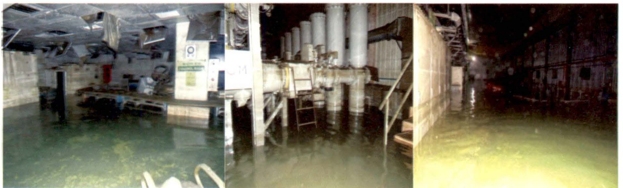
Flooding in Dhauliganga Power House
