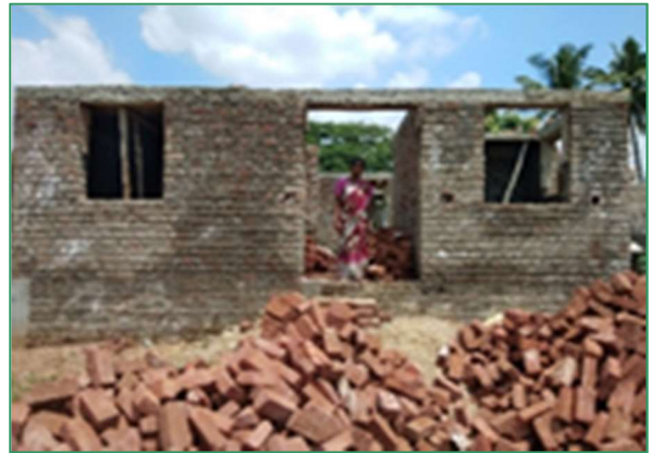
Name: Sumathi (TN1397263), Adiannamalai, house yet to be roof casted shown as completed (Completed and Roof cast on same day)
