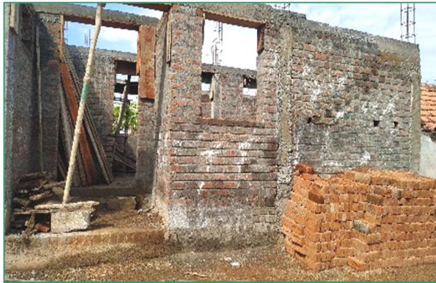
Name: Susei Periyanauyakam (TN1413866), Alaganandal, house yet to be roof casted shown as completed - 24/06/2020
