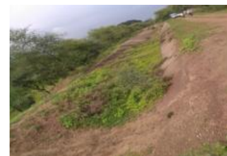
Sliding & silting of lining near Phukujodi village
