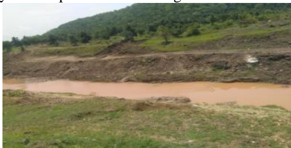
Rock zone in the Canal bed and side at RD 64.5 to 65.5KM of Right Main Canal
