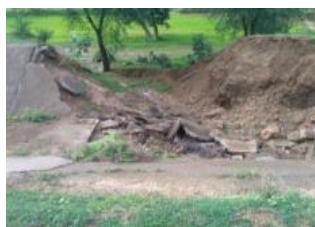
Breach in embankment near Phukujodi village
