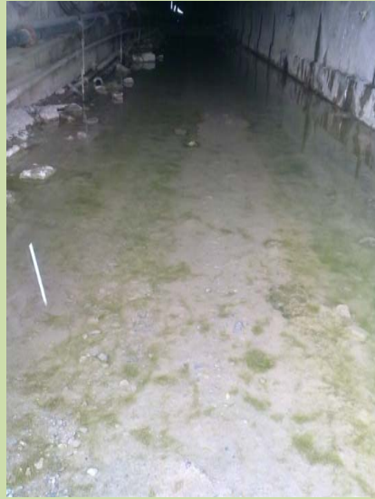
Tunnel T – 1 water logged
