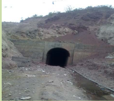
Portal T6 P1, which is unstable
