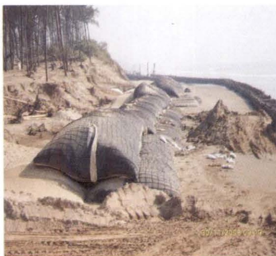
Damaged Geotubes in November 2008
