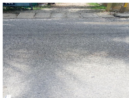
Picture 1: Aggregates stripped off the BC surface of a road in Thiruvananthapuram district (photo taken on 04/10/2018)
