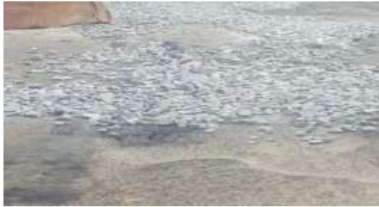
Picture 4: Potholes filled with 36 mm aggregates without cutting the potholes into regular shape (photo taken on 24/09/2018)
