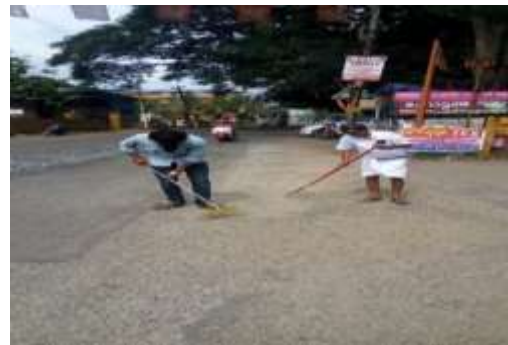
Picture 6: Detached loose aggregates from filled up potholes being cleared by the public due to improper method of construction (photo taken on 24/09/2018)
