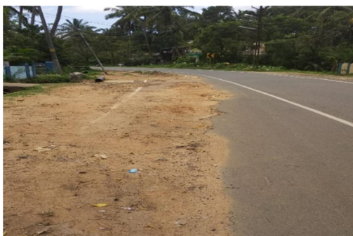
Picture 10: Unattended restoration works after laying of pipelines reduced the width of carriage way(photo taken on 07/09/2018)
