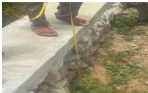
Picture 2: Improperly constructed retaining wall of a road leaning inward in a work in Palakkad district (photo taken on 29/09/2018)
