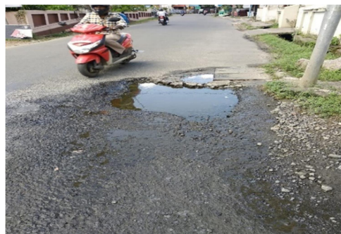
Picture 11: Unattended pipe leakage caused pothole in newly resurfaced road (photo taken on 07/09/2018)
