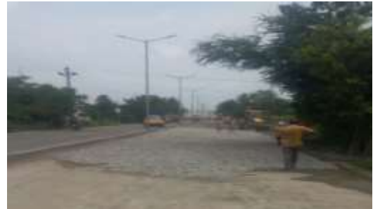
Picture 5: Usage of 36mm aggregate for bitumen levelling course in violation of GOK stipulation (photo taken on 27/09/2018)
