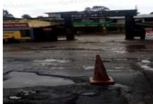
Picture 7: Potholes in front of Taluk Hospital, Thuravur in NH 66
