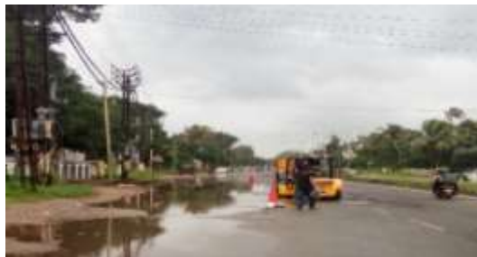
Picture 8: Lack of drainage caused water logging and potholes, reducing the width of carriageway in NH 66 (photo taken on 14/08/2018)
