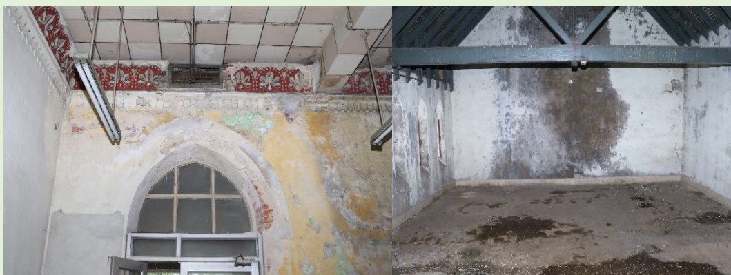
Missing inlay designs
