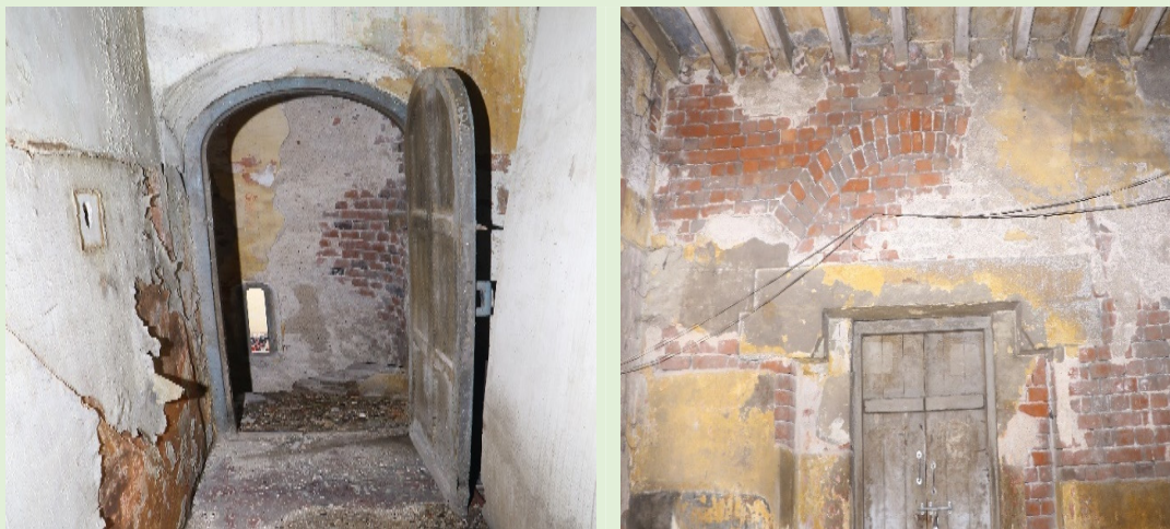
Peeling off plaster
