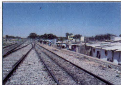
Encroachment in the Safety Zone at Yeshwanthpur Station Yard, Bangalore, South Western Railway
