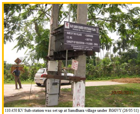
110.450 KV Sub-station was set up at Sandhara village under RGGVY (26/05/11)
