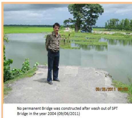
Execution of substandard work of Raha-Barapujia Road (09/06/11)
