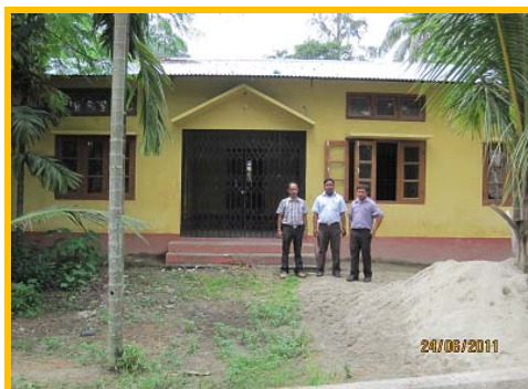
Newly constructed Salmari 2 SC remained unutilised since last 18 months due to want of electrical connection (24/06/11)
