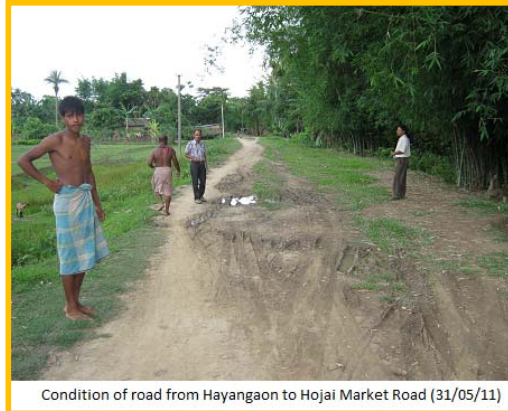
Condition of road from Hayangaon to Hojai Market Road (31/05/11)
