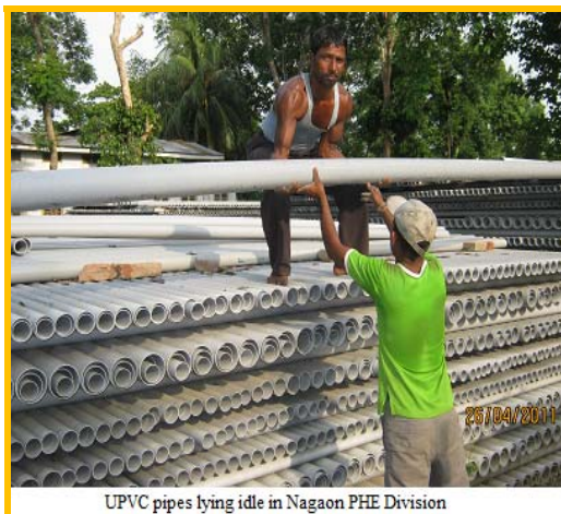
UPVC pipes lying idle in Nagaon PHE Division
