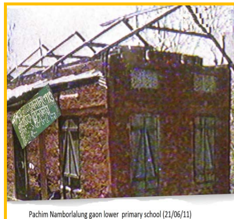
Photograph showing the dilapidated condition of school
