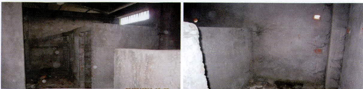
Photographs of Business Center in Dokmoka Town, showing no evidence of any service works being done
