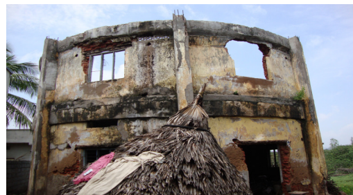
Shelter in dilapidated condition at Dibbavanipalem-2 in Visakhapatnam District
