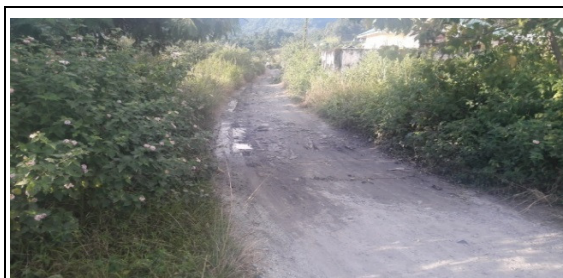
Rural Link Road constructed near Yatri Niwas, Roing executed at ₹ 3.00 lakh in 2018-19 was actually laying of granular materials on the existing road
