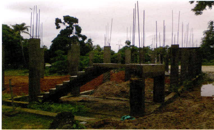
Incomplete building for outpatient in MCH, Alappuzha.
