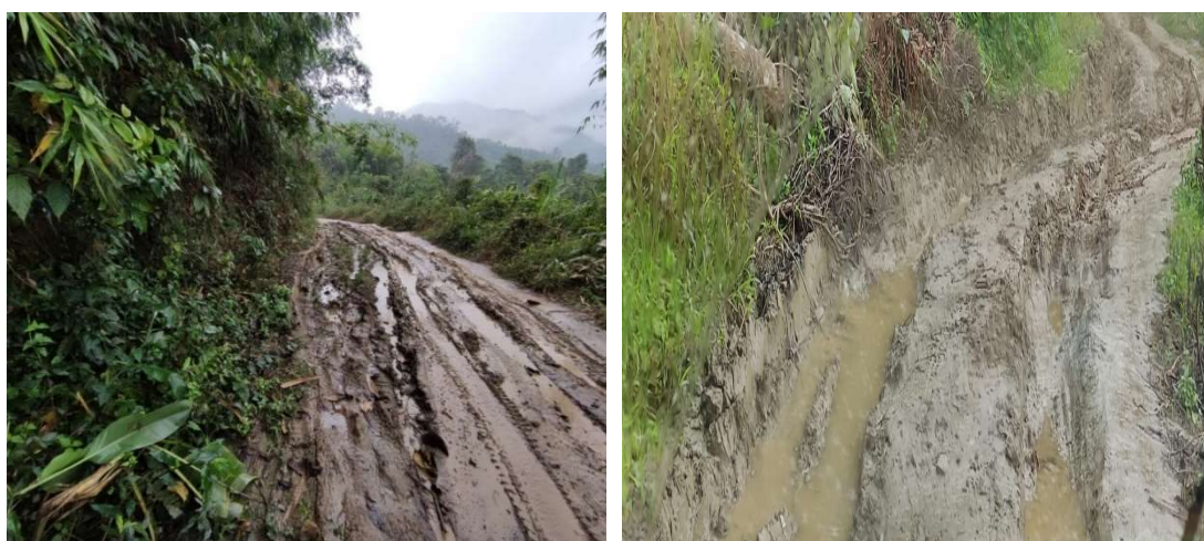
Pic: Link-road without side drain and gravel Pic: Link-road without side drain and gravel
