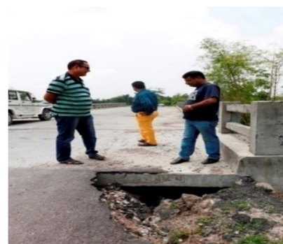
Embankment Failure of RCC Bridge No. 16/1 on Dotoma to JogdoiMusalmanpara road. (Photograph Taken on 3 June 2018)
