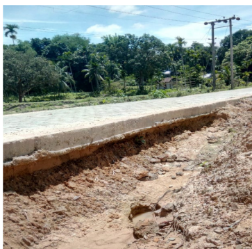
Photograph (12 July 2018) of eroded base course due to non-construction of sub-surface drain in the Irongmara to Silcoorie Road under Sílchar Rural Road Division.
