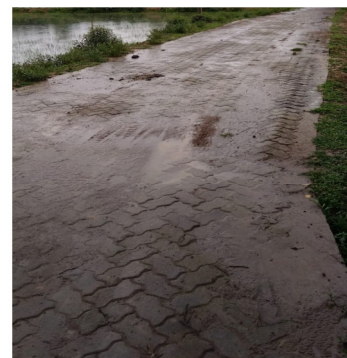
Photograph (27 June 2018) of undulating road surface of the road Pioli Phukan road under Charaideo Rural Road Division, Sonari.
