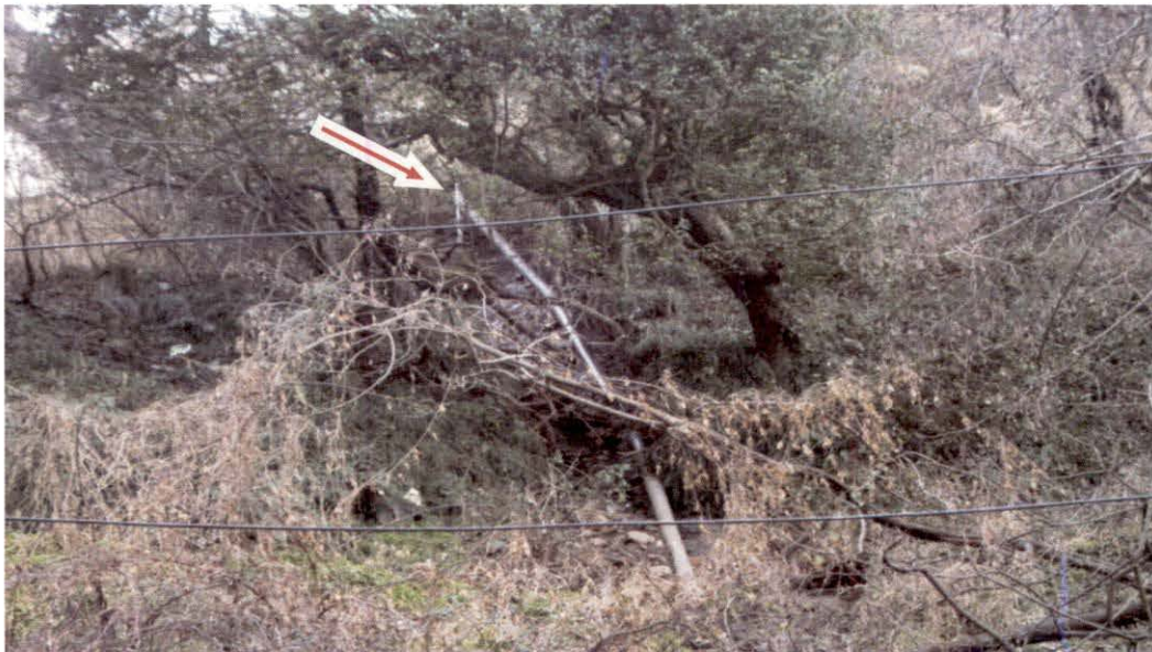
Missing link of sewer line adjoining IGMC & Hospital (8 February 2011)
