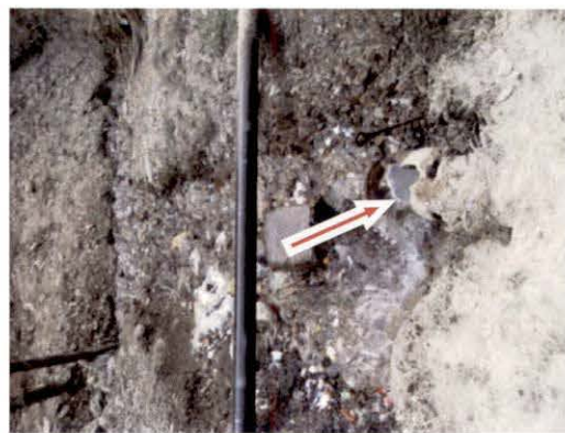
Broken sewer line below IGMC & Hospital (8 February 2011)
