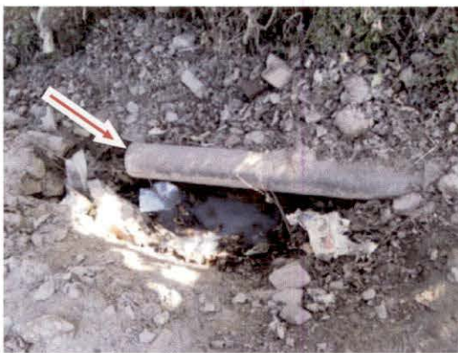
Missing link of sewer line between Vikasnagar-Panthaghati area (8 February 2011)
