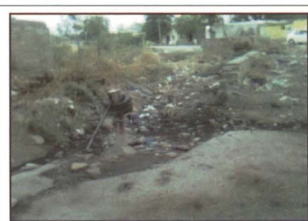
Hand pump in the middle of heap of waste (Udanoor village, Kalaburagi district) 20.03.2014
