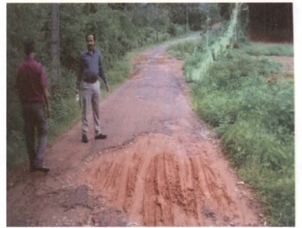
Condition of asphalted road within six months of construction in Aivathoklu village (Dakshina Kannada) (16.07.2014)
