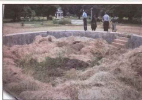
Waste material (dried grass, etc.) dumped in the fountain pool at Kuppanna Park, Mysuru (19.06.2014)
