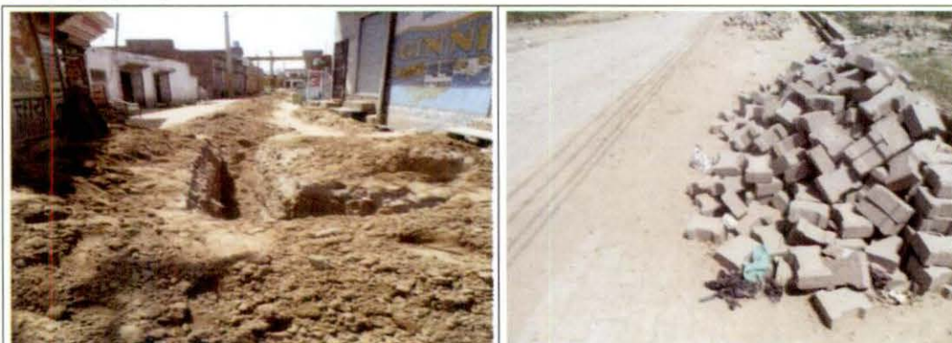
Interlocking Paver Block street damaged by PHED for laying of Sewer in ward 5 and 12, Ratia (10 April 2013)
