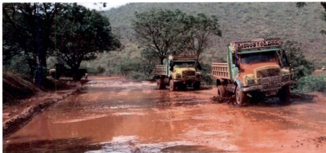
State Highway-49 Road in Sandur area damaged by mine lorries
