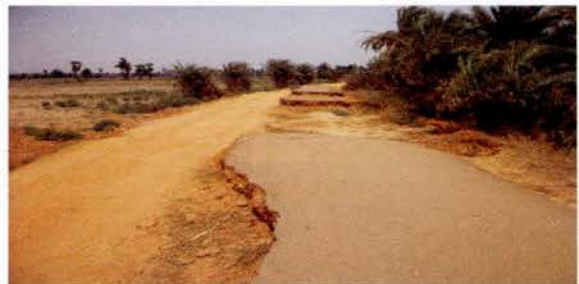
Bipulingi to Gangapur road fully washed and not restored
