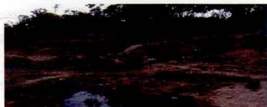
Embankment in Subarnarekha River not restored
