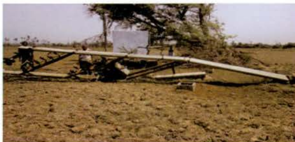
LIP at Agasti Nuagaon-1 village under Chhatrapur Block not restored
