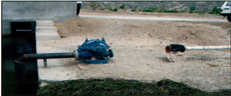
Photograph showing non-connection of rising main of water supply scheme with source (06.07.2010)
