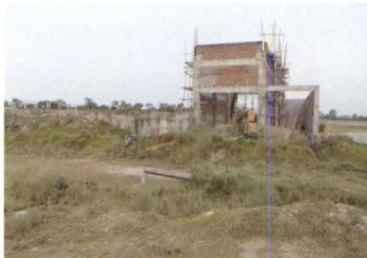
Incomplete SHP at Mathauli
