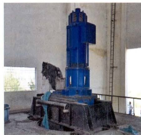
Turbine of incomplete work at Tejpura SHP
