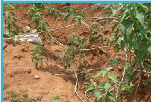
Work ID: 030312020024050029 GP/Mandal/District: Gunnempudi/Butchayapeta/Visakhapatnam Expenditure incurred: ₹24,49,785 Sluice completely closed due to soil erosion, defeating the very purpose of irrigating the ayacut
