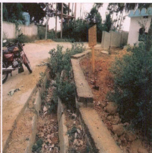
Abandoned work of construction of compound wall of graveyard in Beechaganahalli GP (18 May 2012)
