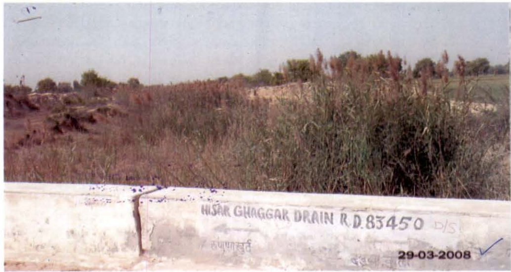
Non-functional Hisar Ghaggar drain at RD 83450
