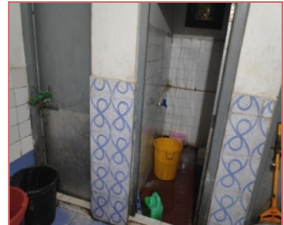
Damaged & Non-functional Toilets
