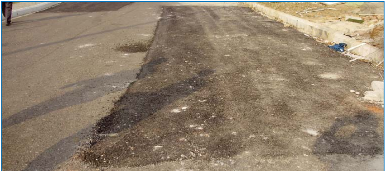
Patched up in road surface
