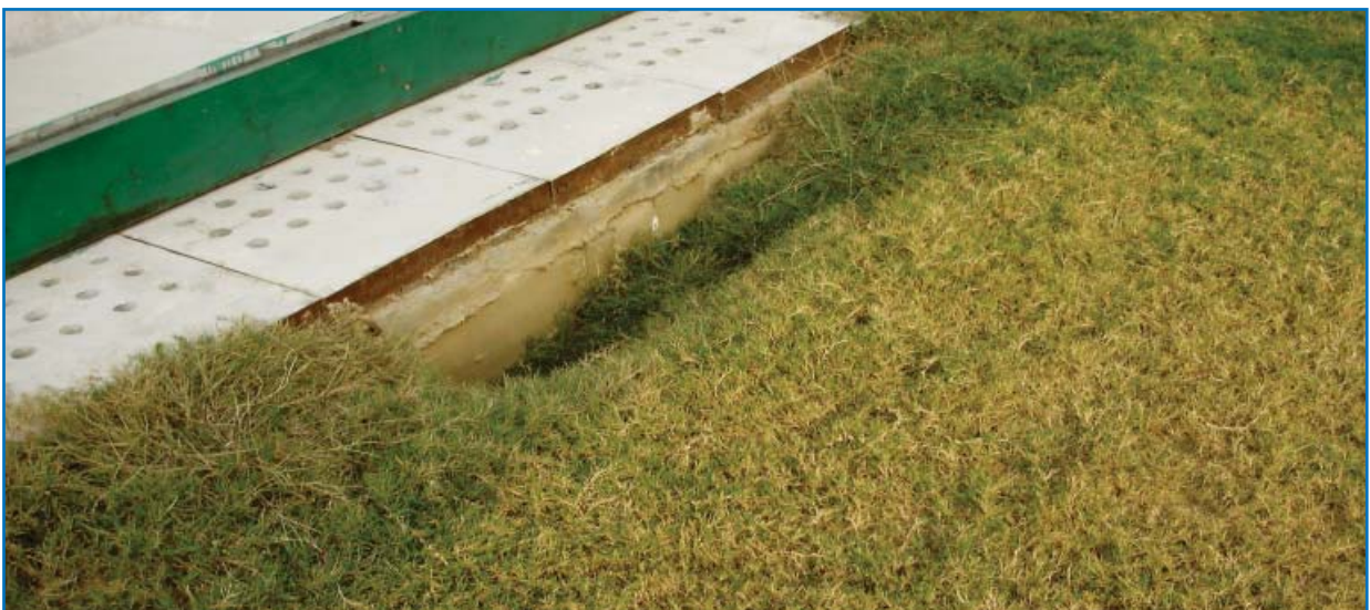
Weepholes in target area
