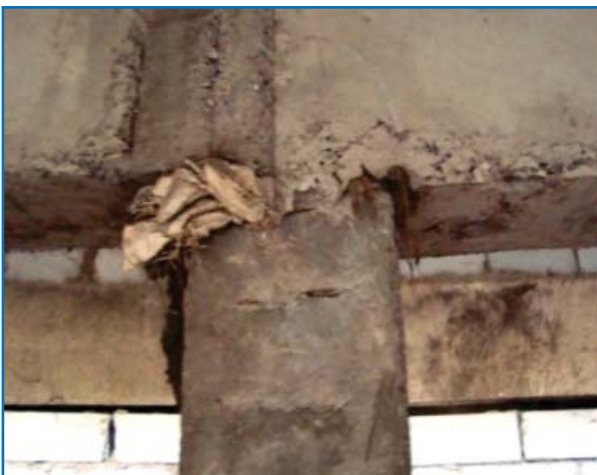
Plastic Bag in Beam and Shear Wall Joint (- Report No. 9-Tower-15)
