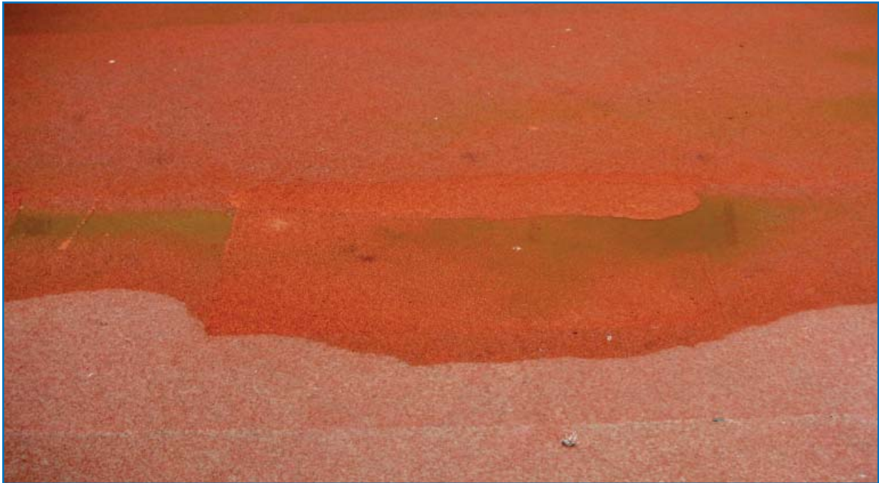
Patches of water logging
