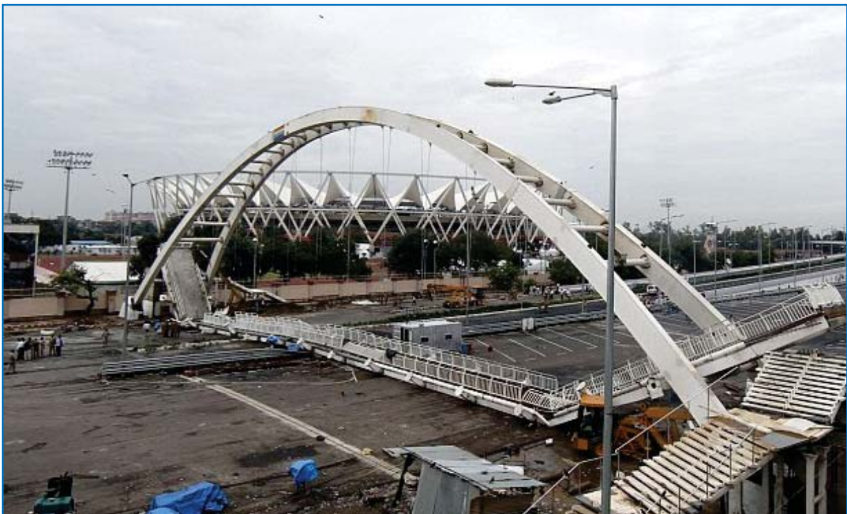
Collapsed FOB near JLN Stadium
