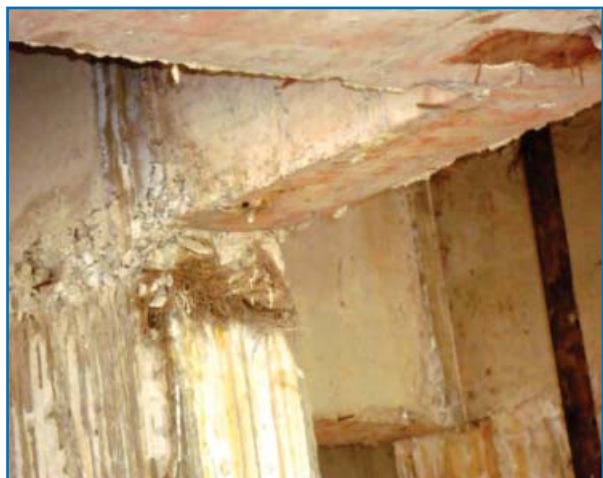
All in one (honey combing, seepage, corrosion, and jute bag) in Tower 7 as reported in CBRI Report No. 9
