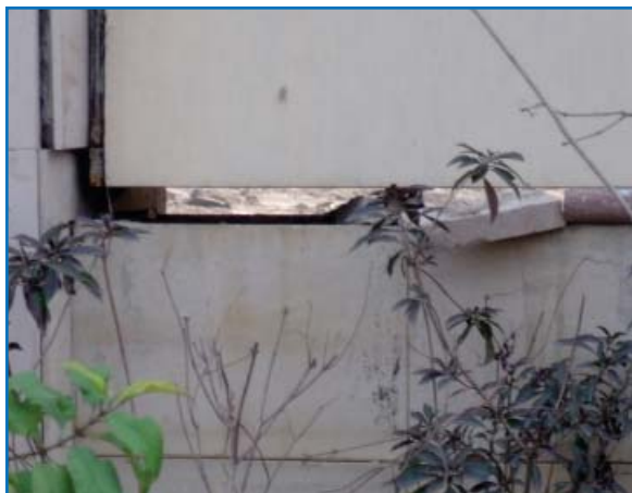
Unfilled Gaps in boundary wall
