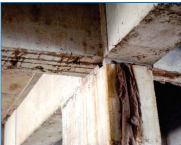
All in one (Exposed Steel, Hole in Beam Column Junction, Insertion of Jute Bag) Tower 15 as reported in CBRI Report No. 9
