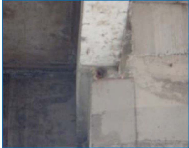
Half the width of the beam is outside the column - Report No. 3
