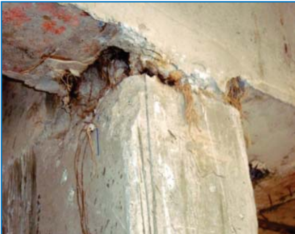
Chidiya Ghar in Beam-Column Joint (- Report No. 9 -Tower-5)
