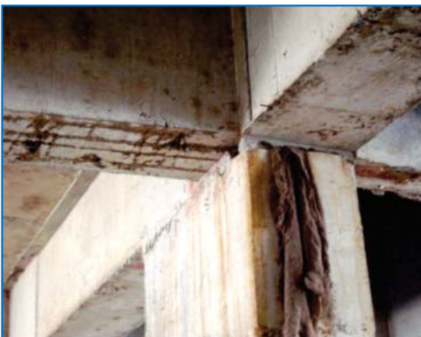
All in one (Exposed Steel, Hole in Beam Column Junction, Insertion of Jute Bag) Tower 15 as reported in CBRI Report No. 9
