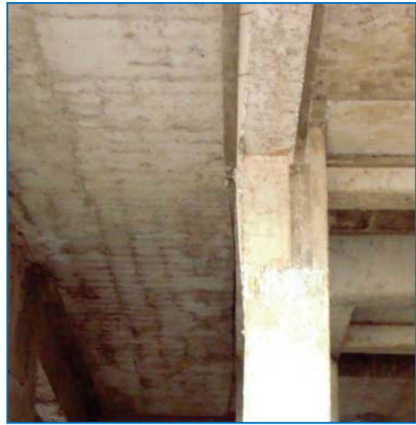
Two in one: Tilt of the column and lack of cover for the reinforcing steel (Tower-34, Upper Basement) Report No. 9
