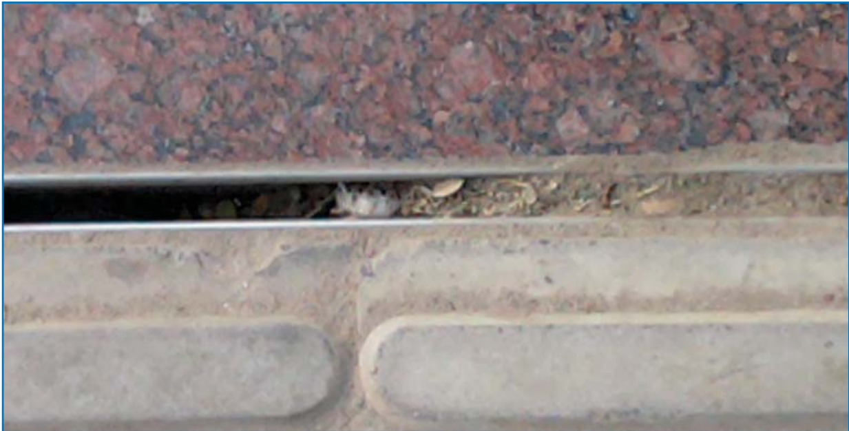
Choked polymer drain
