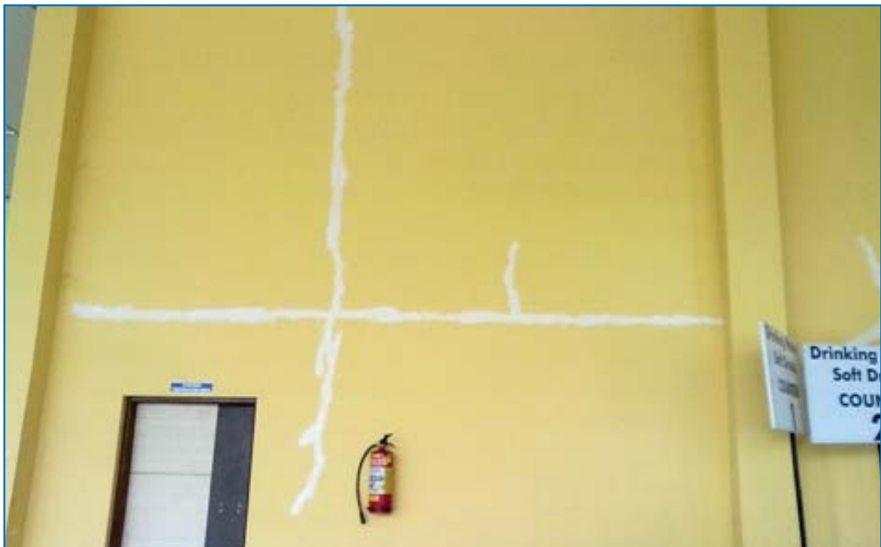
Badminton hall with cracks on the wall
