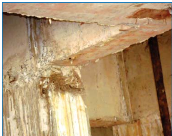
All in one (honey combing, seepage, corrosion, and jute bag) in Tower 7 as reported in CBRI Report No. 9
