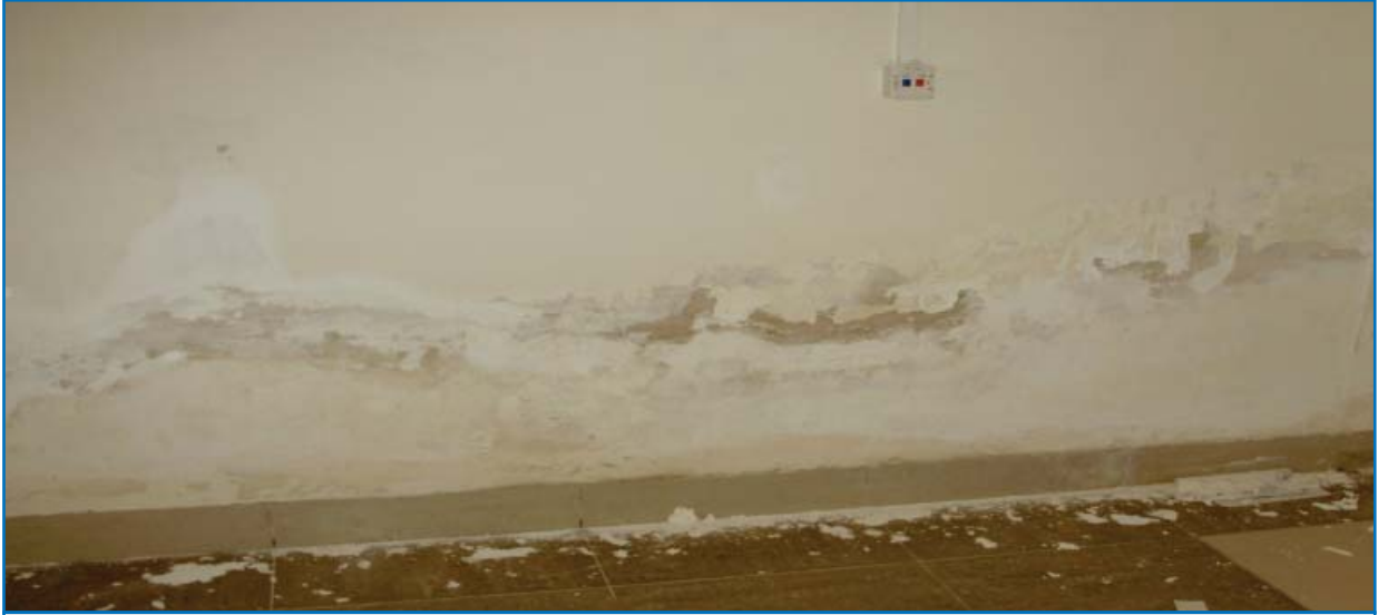
Seepage in walls
