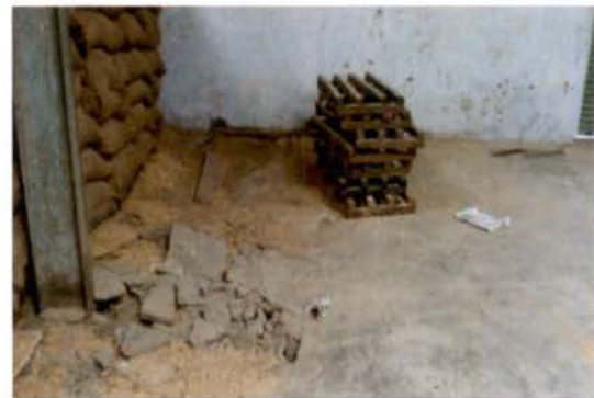
Poor condition of warehouses at Raichur – July 2015
