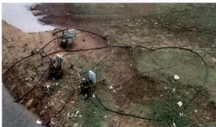
Photo showing an unauthorised IP connection (including motors and portable transformers) – dated April 2015
