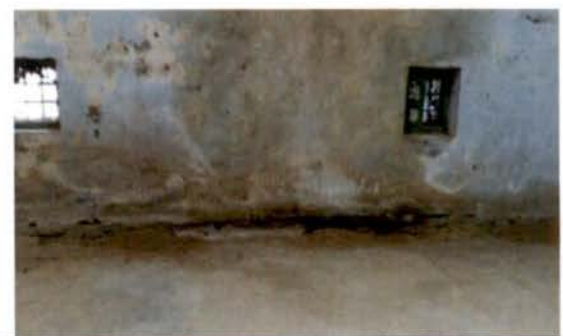
Water seepages and damaged floors at Raichur-July 2015
