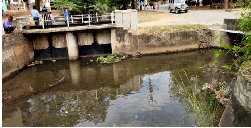
Figure 3: Water seepages due to damaged shutter
