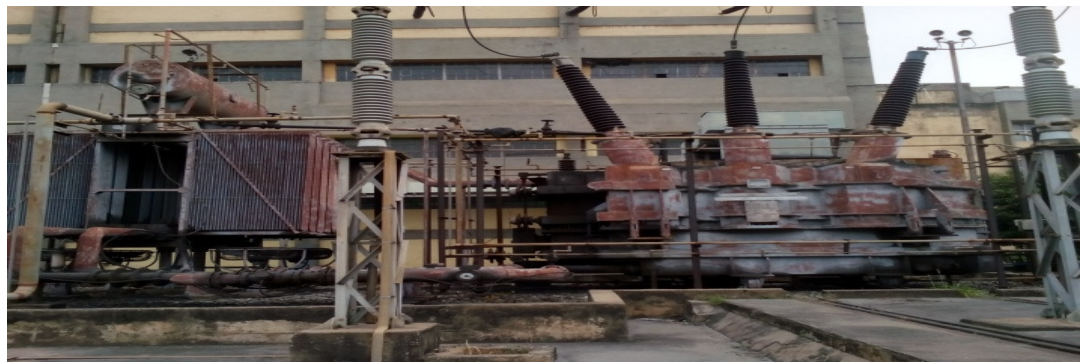
Unit Auxiliary Transformers lying unutilised in TTPS
