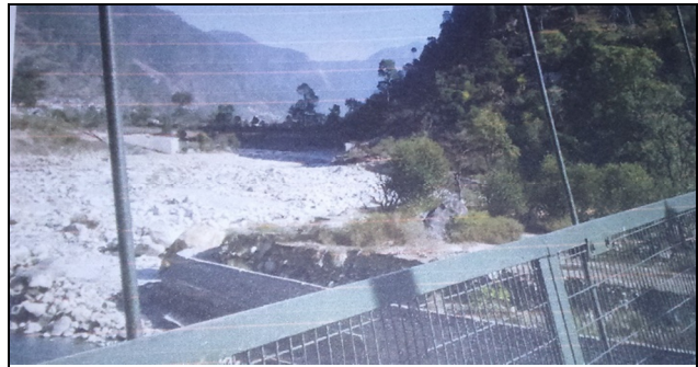
Photograph (taken from newly constructed bridle bridge) showing sites of both bridges at Nakuri and collapsed Motor Bridge which is being constructed 100 metre distance in upstream.
