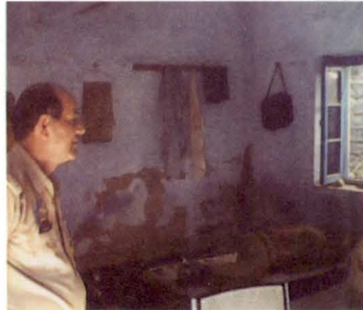
Bad condition of Police station Nowshera
