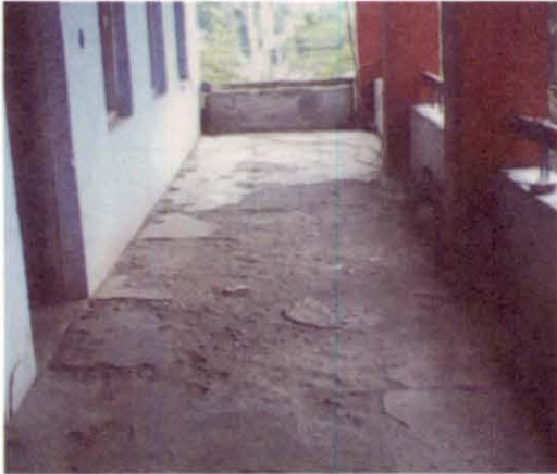
Damaged flooring of Police station Rajouri
