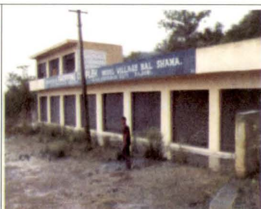
Vacant shopping complex, Balshama, Sunderbani
