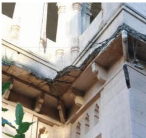
Picture 2 Dilapidated condition of Darbhanga Hall
