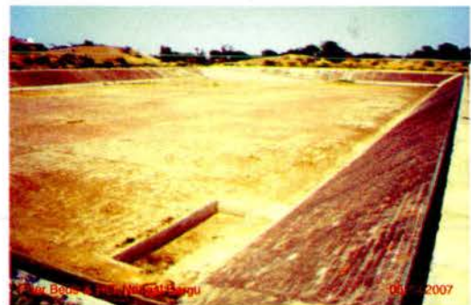
Empty storage and sedimentation tank at Nangal Dargu water works
