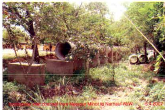
Incomplete inlet channel from Neerpur Minor to Narnaul water works
