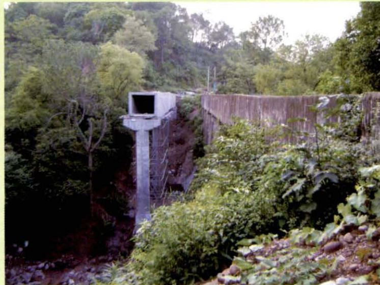
Aquaduct at kms 6.867 to 6.909 kms lying incomplete due to slow pace of work by the contractor
