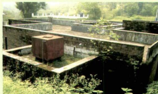
Dilapidated condition of residential facilities for staff CHC Bhota
