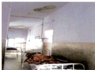
DH Mavelikkara- Exposed ceiling in Paediatric Ward - 11 June 2013
