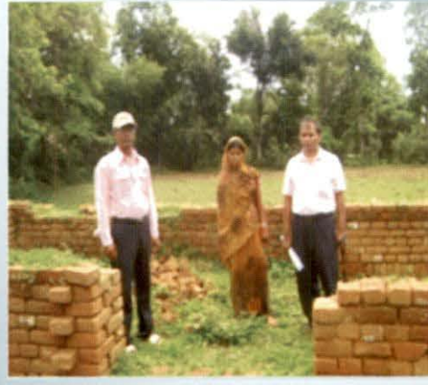
IAY house in scheme No. 115/2010-11 at Forest Block GP in Gurabanda block of East Singhbhum district abandoned after ₹ 48,500 (final payment) was paid to the beneficiary.
