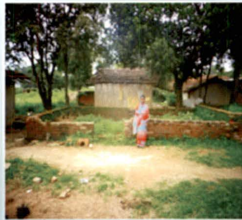
IAY house in scheme No. 88/2009-10 at Hurhuri GP in Ratu block of Ranchi district abandoned after ₹ 35,000 (final payment) was paid to the beneficiary.
