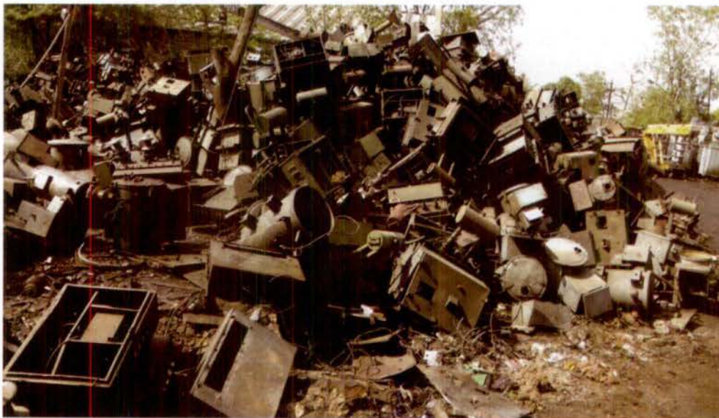
Failed transformers lying in heap at JPDC ACOS
