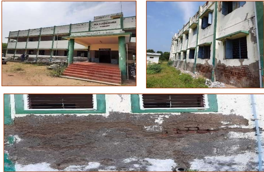
Exhibit 4.9: Poor quality of construction - Images of Government High School, M.Nedungulam, Ramanathapuram district
