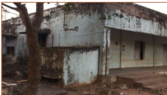
Exhibit 4.5: Classes held dilapidated building at GHSS, Sirugramam, Cuddalore
