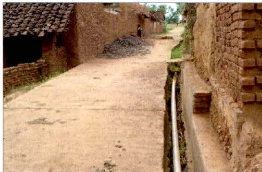
View of pipeline laid in existing drain of cement concrete road in village Khamha for which cutting of cement concrete road was shown. (Spot: main road Khamha village, August 2009)
