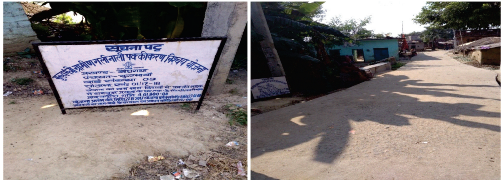
Construction of PCC road without drain in ward no. 9 of GP Kurmawa (Gaya); Scheme no.- 01/2017-18
