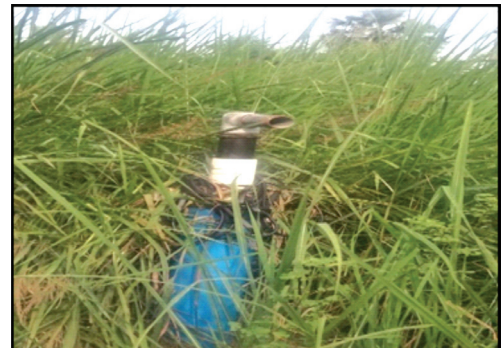
Water supply works taken under MMGNPY were left abandoned after boring work. (Ward no. 05 of GP Gahar Pachhim, Samastipur); Date-30 August 2018
