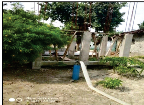
Water supply works taken under MMGNPY were left abandoned after boring work. (Ward no. 09 of GP Gangsara, Samastipur) Date-30 August 2018
