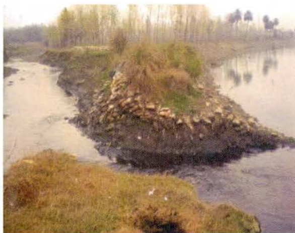
Washed away portion of ditch drain polluting water of Western Yamuna Canal
