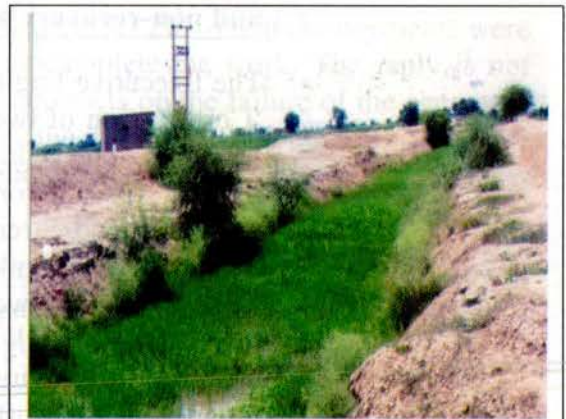
RD 96000 Rangoi Kharif Channel showing silt/ grass on Recharge Well
