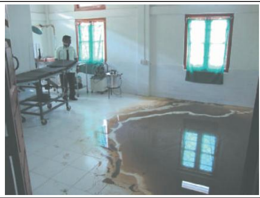
Operational Theatre - not used and full of dirty water
