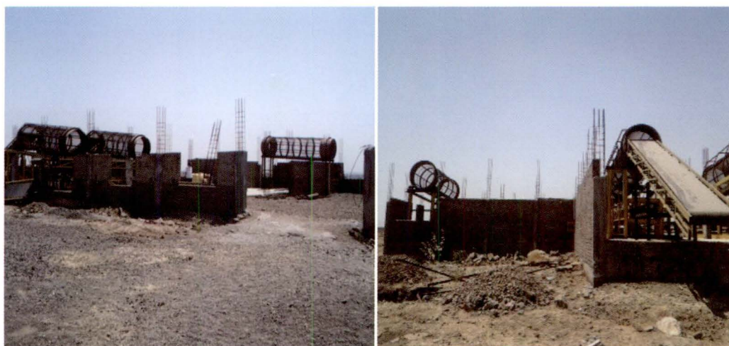
Waste processing facility in Jalna, Maharashtra
