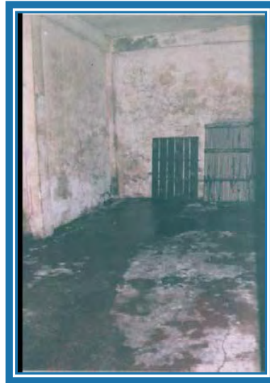
Mawlongghat, Shillong - Dilapidated Godown
