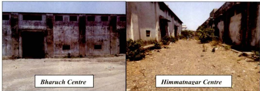
Picture 3.2: Showing poorly maintained Godowns
