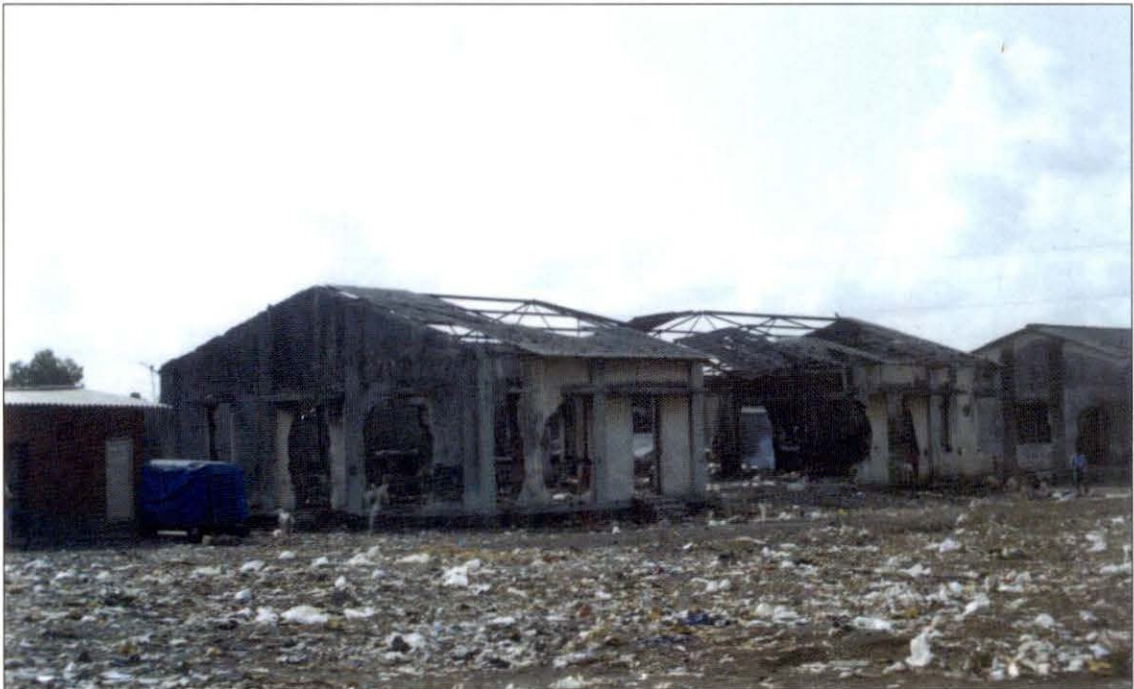
Paragraph 3.9.5.4.2 : Government hostel barracks at Chembur, Mumbai being used for dumping garbage
