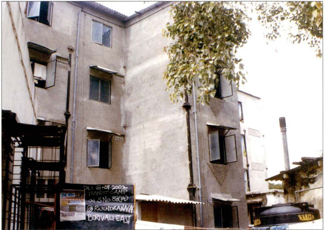
Paragraph 6.17 : Multi storeyed RCC structures constructed on the land allotted for construction of transit tenements
