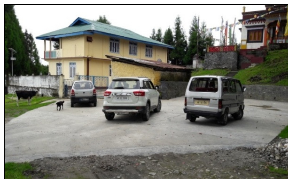
CC platform constructed instead of playground in the middle of an approach road to a private residence.
