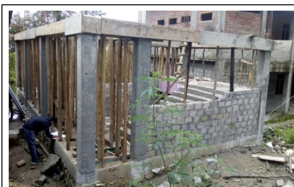
The status of the work 'Rostrum at Seru Secondary School' shown to have been completed in March 2017.
