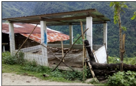
Bus Waiting Shed at Row Village enclosed with sausage wire being used as store room.
