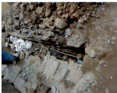
Work held up due to non-shifting of underground utilities by PHE, BSNL. (Jammu & Kashmir)
