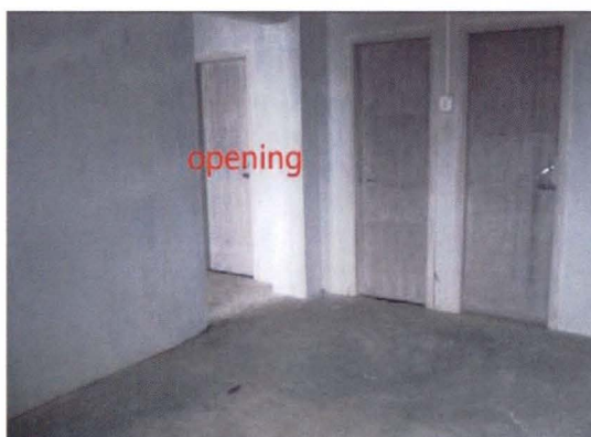
Nagaland- BSUP project, Kohima: Two DUs with opening on the adjoining walls – Photo taken on 03/06/2011
