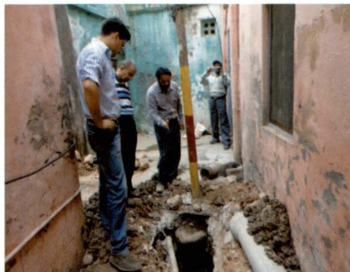
Work held up due to non-shifting of electric pole by Power Development Department (Jammu & Kashmir)
